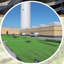
屋上緑化 Rooftop greenery
