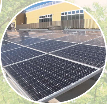
太陽光発電設備 Solar power generation equipment
