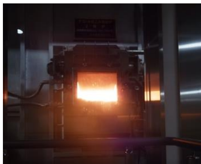
Incinerator Observation Window
