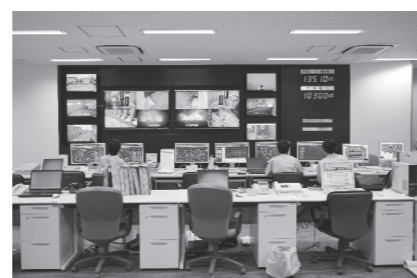
Central Control Room (Nerima Incineration Plant)
